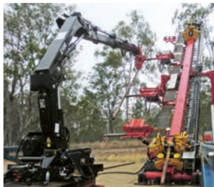
Drill pipe crane with drill pipe gripper and remote control
